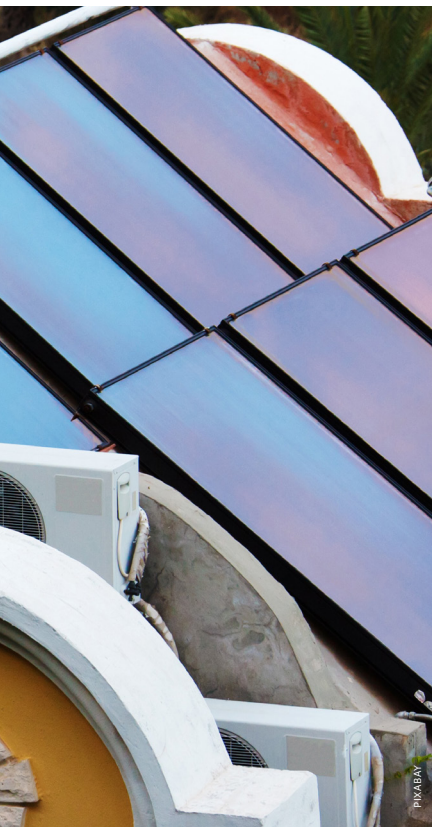
Solar thermal panels on a roof
